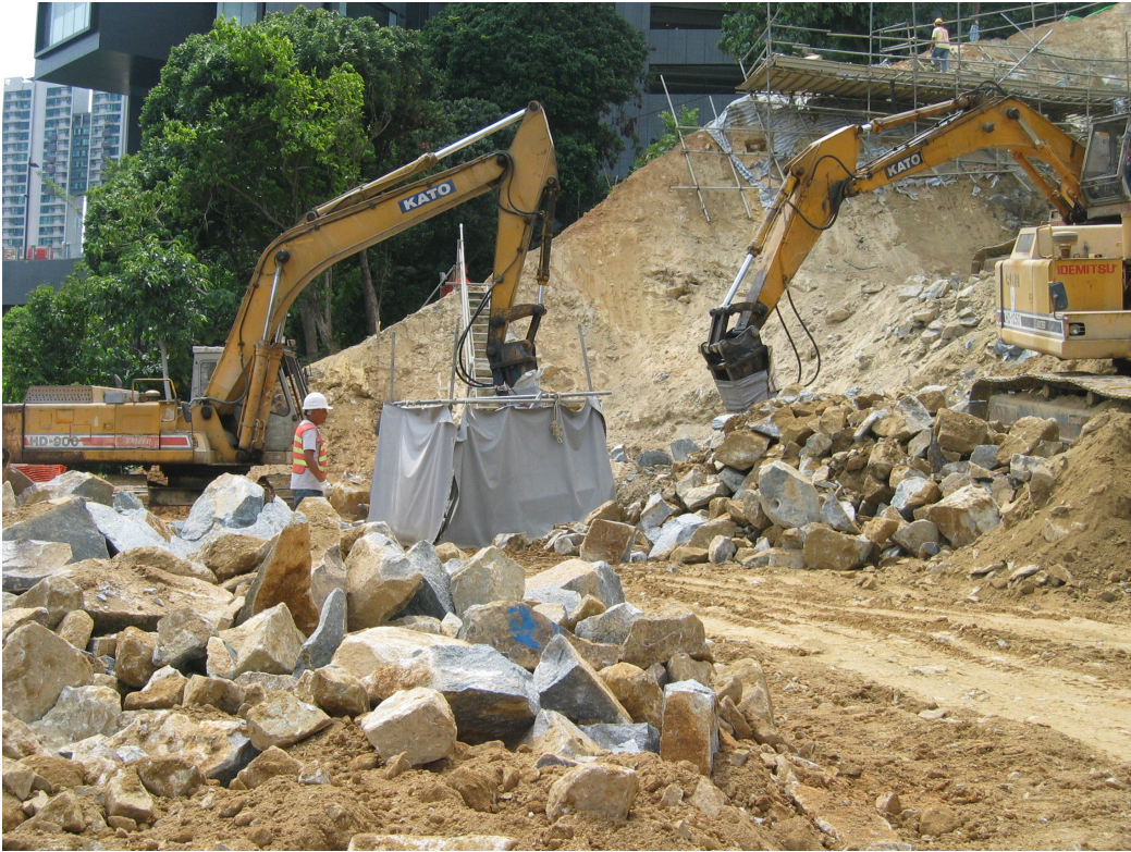
2. Sound insulation sheet surrounding the rock breaking activities as far as possible.
